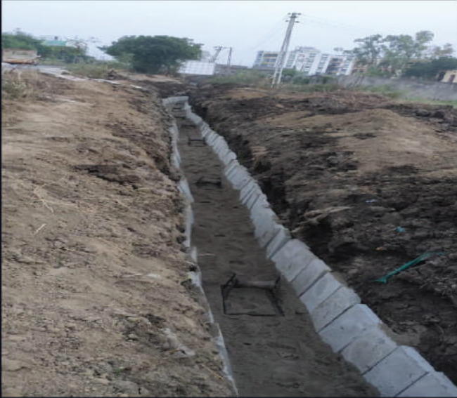
66 kv Thavar – Malhotra ug line
