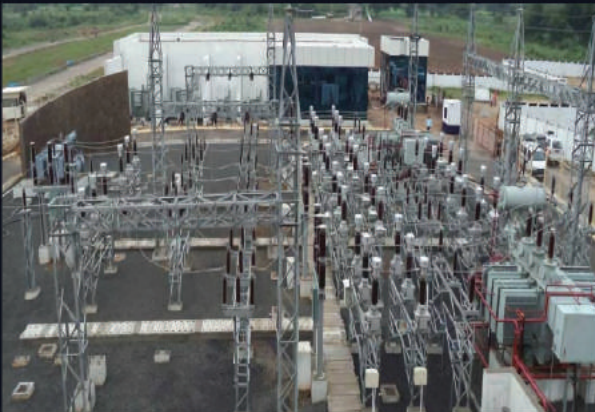
Equipment and scheme testing of switchyard and distribution network
